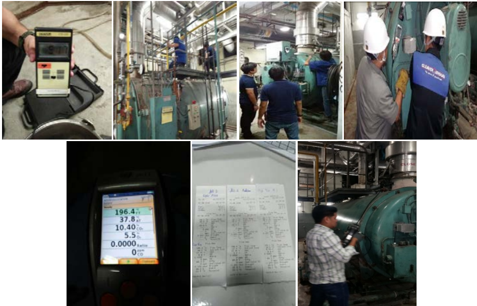
Figure 1 The measurement of boiler operations
