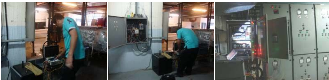
Figure 5 Electricity measurement of heat pump when producing hot water
